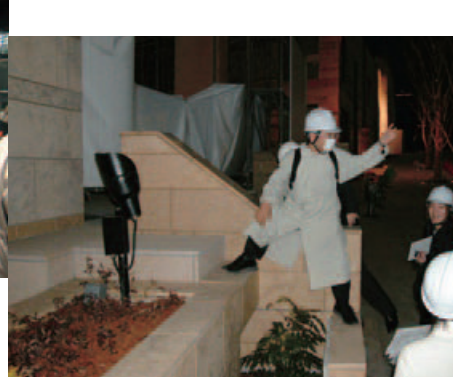
21. けやき坂通りに面した建築外壁の照明。来るはずの大きな樹木が来ないため、照明器具が丸見えである。取り急ぎパイプのカットを指示。 21. Giving instructions for pipe cutting work on lights for the exterior walls of a building on Keyakizaka Dori, which have been left exposed because the trees to be planted around them have not arrived.
