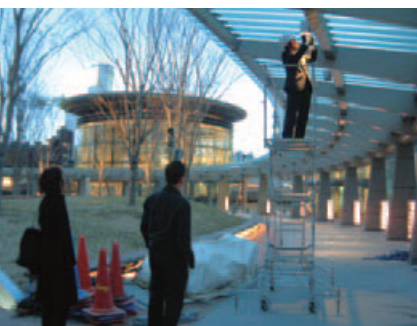
25. Adjusting the lights in the canopy of the 66 Plaza. The distribution of light does not form a seamless belt because the lights are not fitted with spread lenses. We order the lenses to be fitted in time for the opening.
